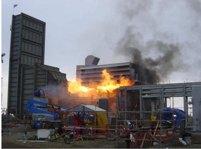
Figure 2. The Calpine Wolfskill Energy Center gas blow incident
