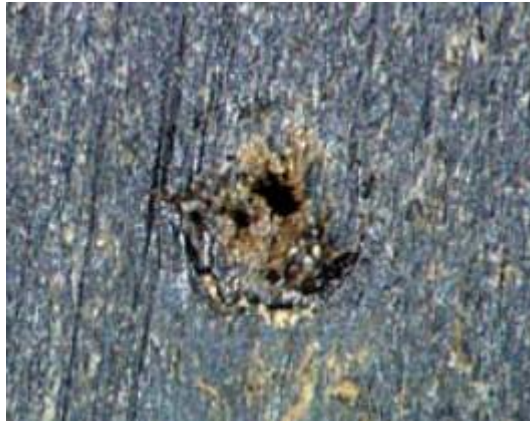
Interior pinhole of damaged pipe
