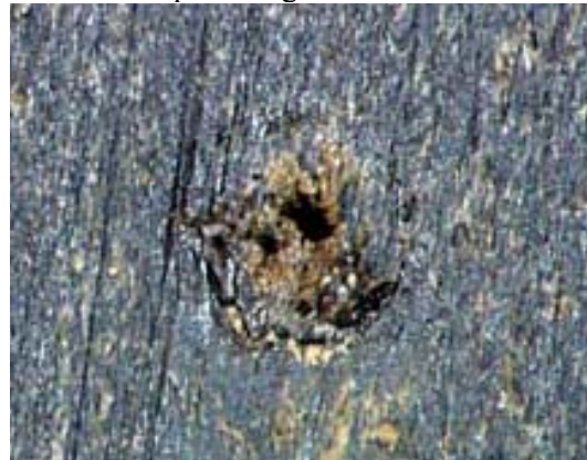
Interior pinhole of damaged pipe
